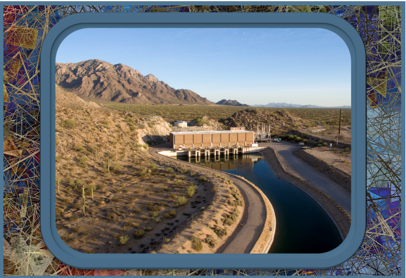
CAP Picacho Pumping Plant
