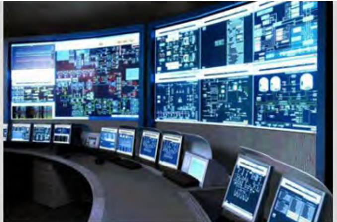
Scada replacement at Control Center
