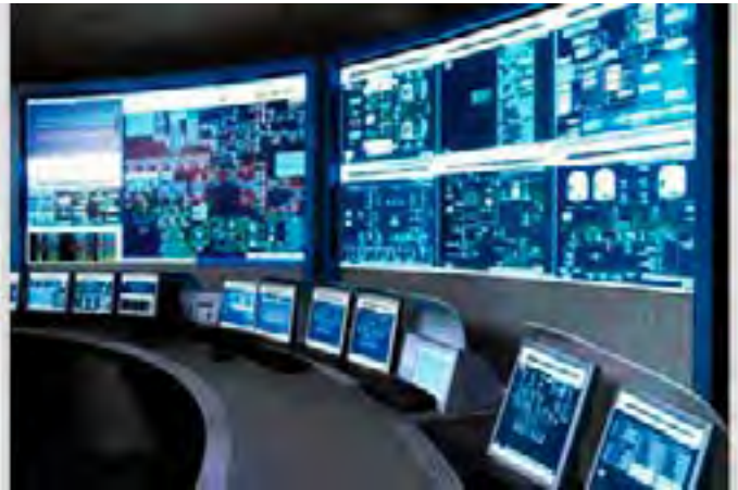
Scada replacement at Control Center
