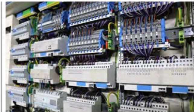
Programmable Logic Controller (PLC) Replacements
