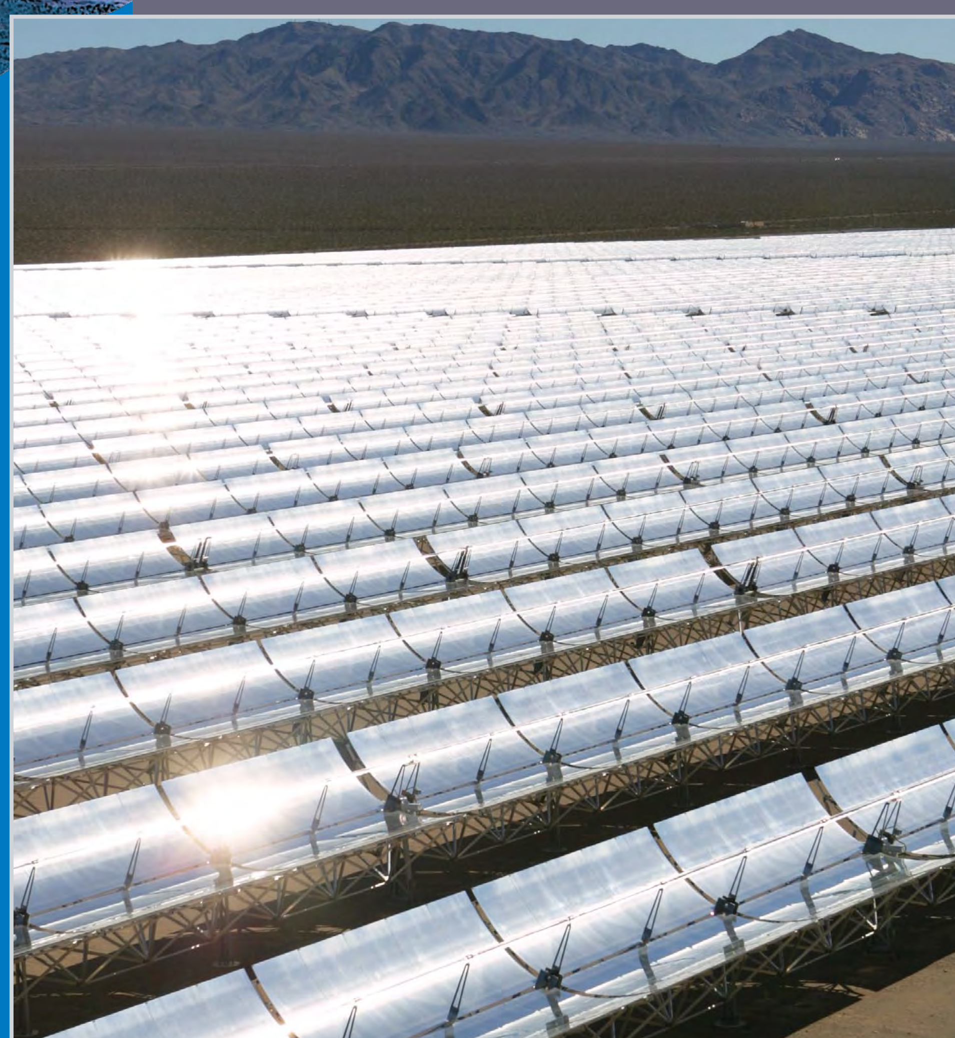
A section of the parabolic troughs from the Nevada One project tracking the sun.
