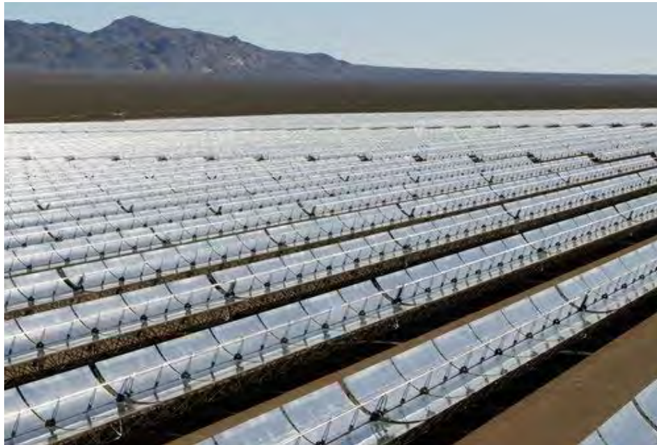
Figure 5. The Nevada Solar One CSP trough system came online in 2007
