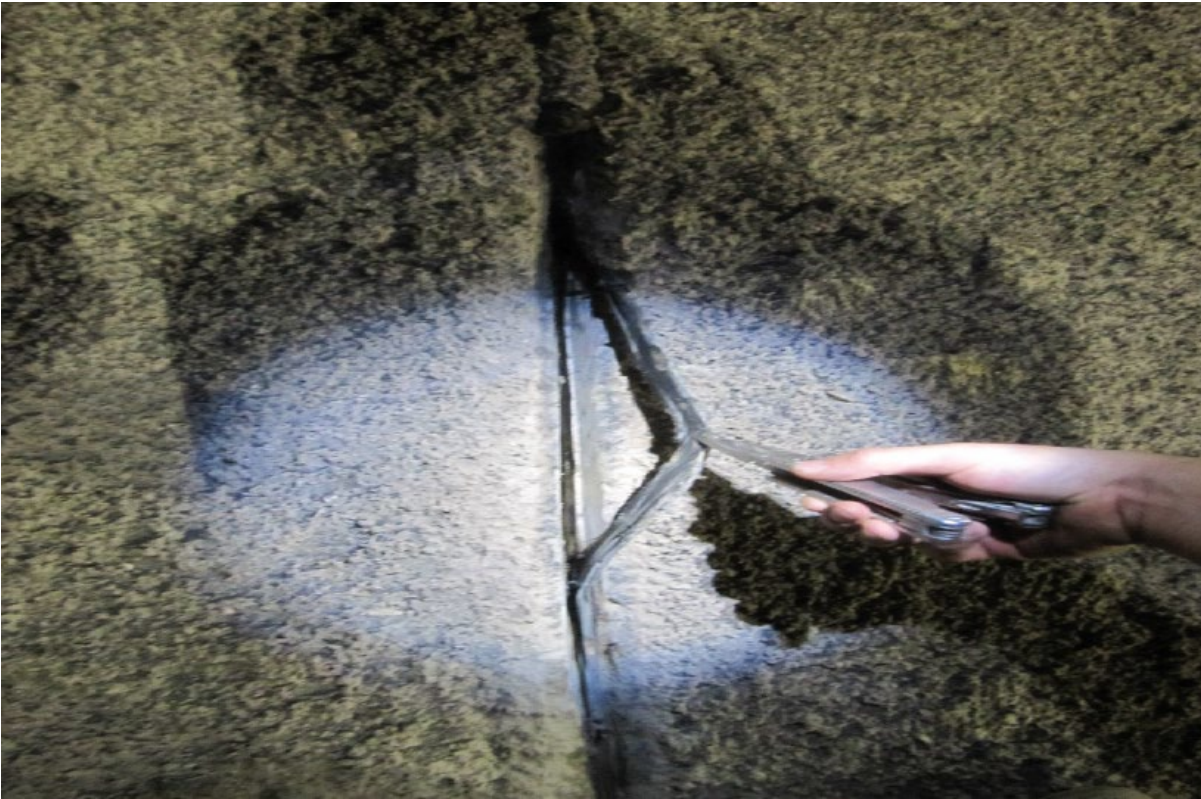
FAILED JOINT SEALING SYSTEM
